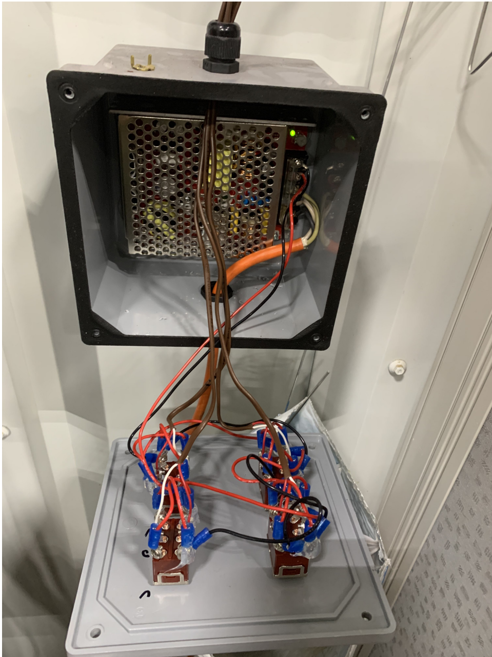
Figure 8: Current Vent Controller (Interior)
