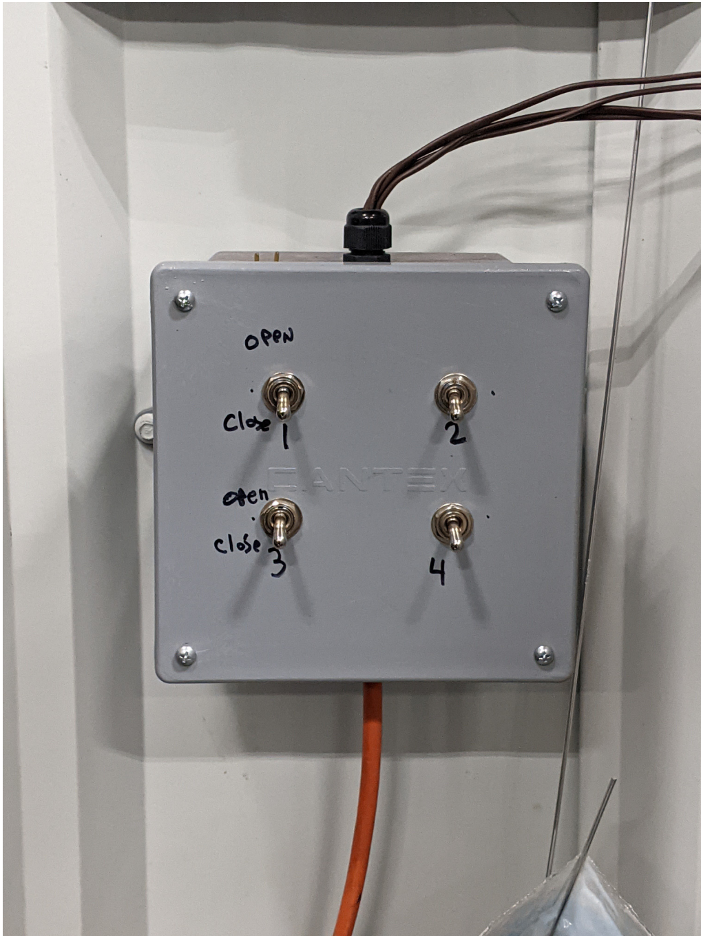
Figure 2.7: Current Vent Controller (Exterior)
