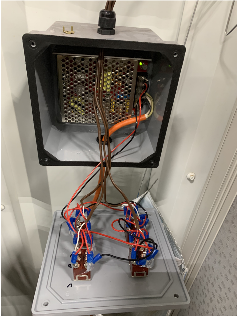
Figure 8: Current Vent Controller (Interior)
