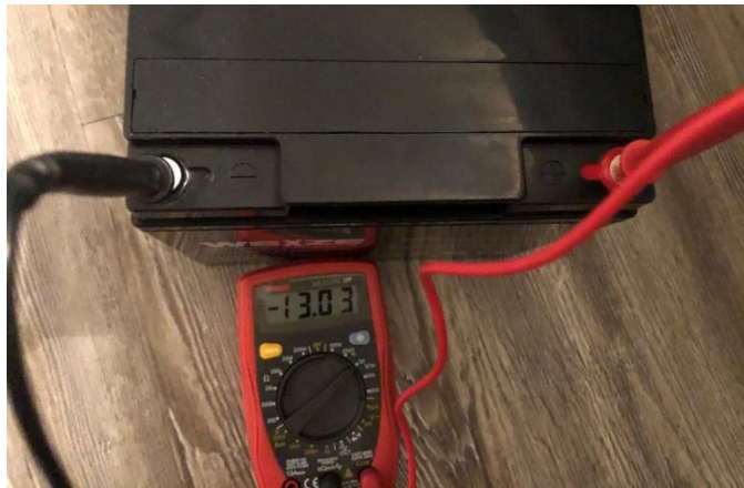
Figure 69: Voltage Testing of the Battery
