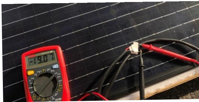
Figure 70: Solar Panel Voltage Testing
