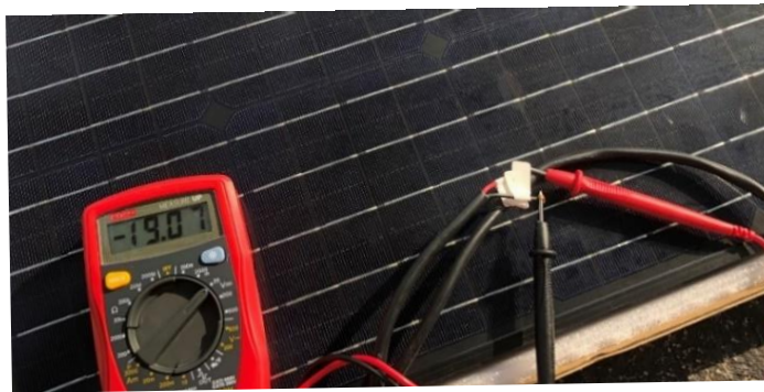
Figure 69: Solar Panel Voltage Testing
