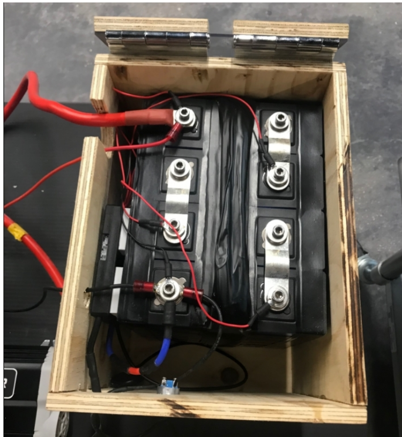
Figure 88: Battery Enclosure Top Down
