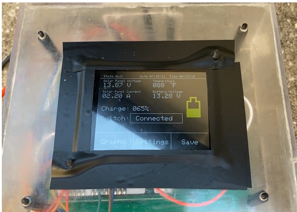
Figure 108: Solar Charge Controller in Custom Enclosure
