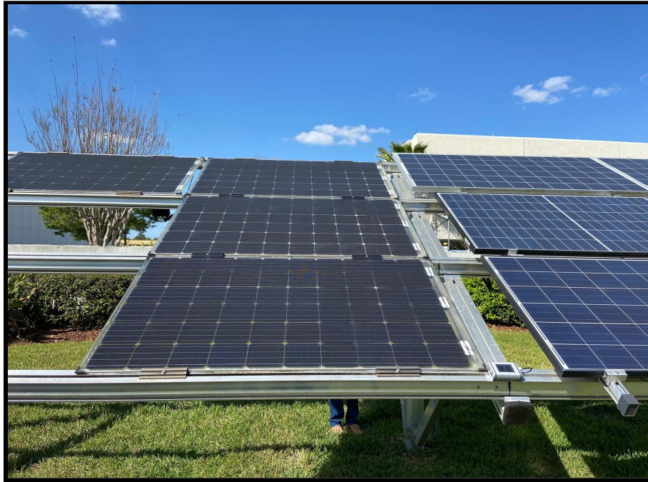
Figure 14: OUC Solar Research Array in Pershing, Orlando
