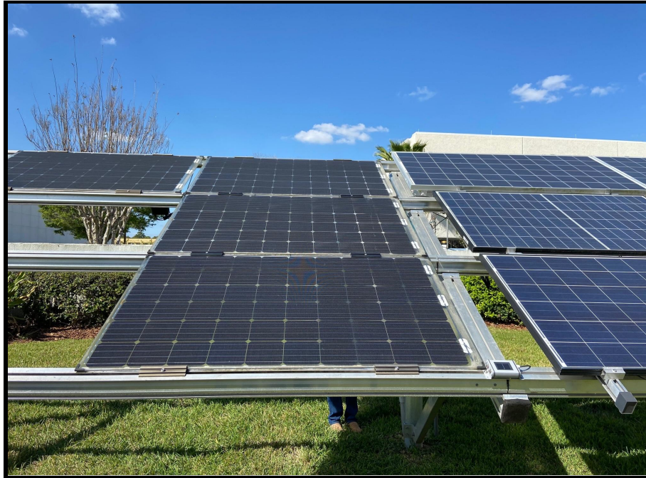
Figure 14: OUC Solar Research Array in Pershing, Orlando
