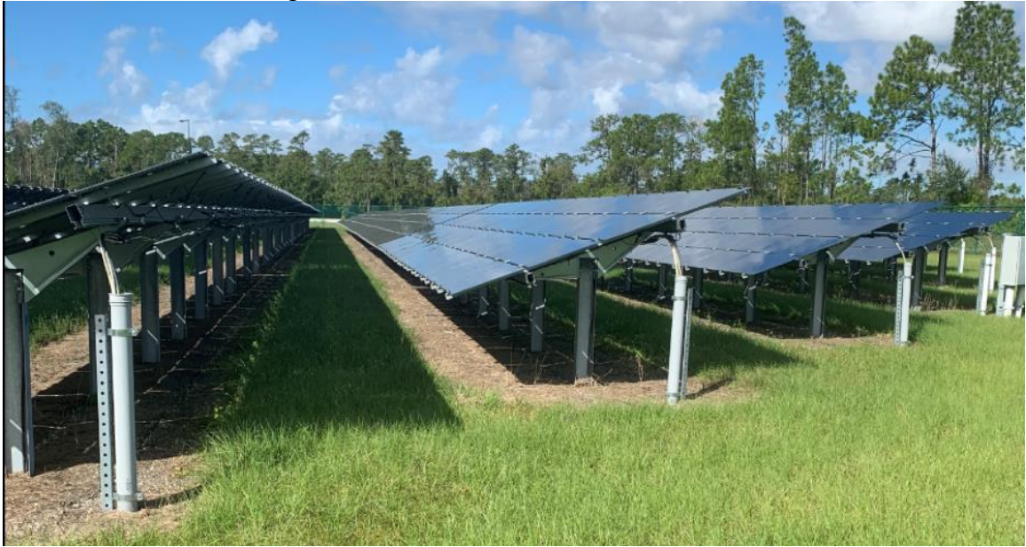
Figure 1: Duke Energy Solar Farm
