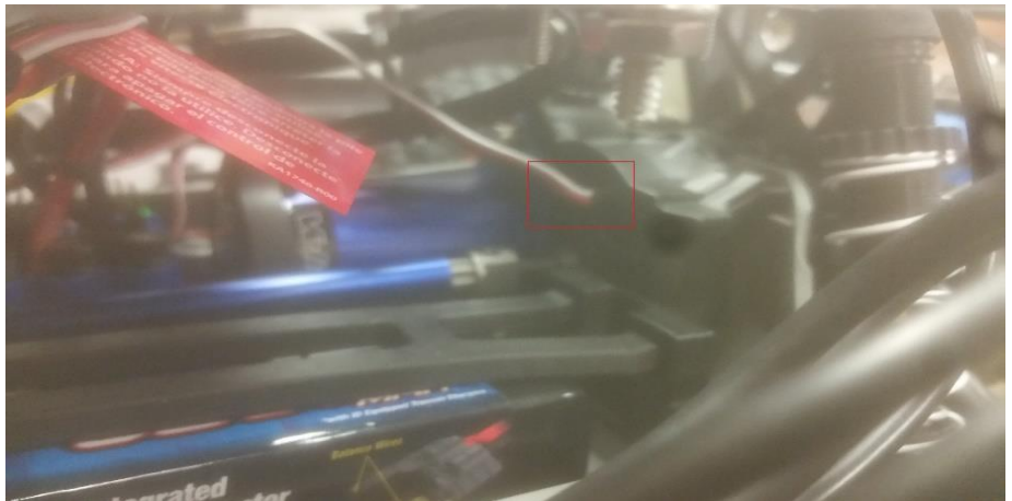
Figure 54- Installed Hall Effect Sensor
