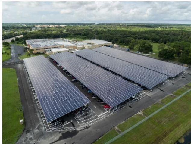
Fig. 1. Solar Panels at Lockheed Martin Parking Lot
