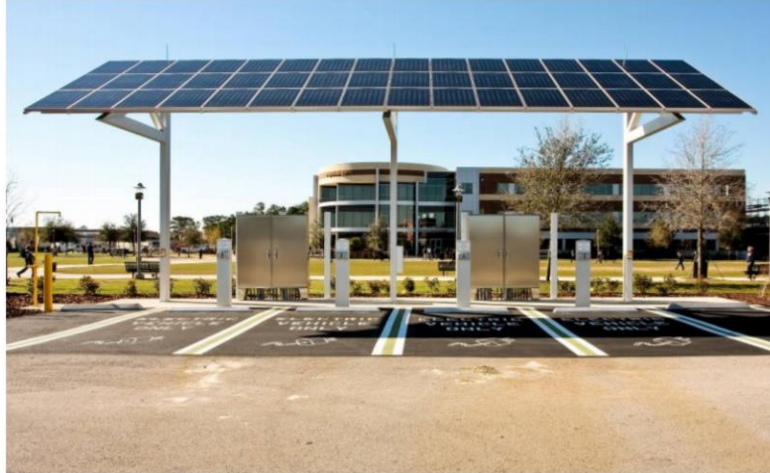
Fig. 3. Solar panels at UCF parking lot
