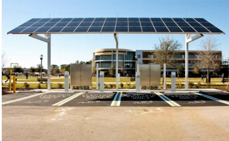
Fig. 3. Solar panels at UCF parking lot
