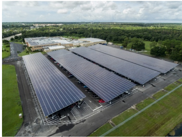
Fig. 1. Solar Panels at Lockheed Martin Parking Lot
